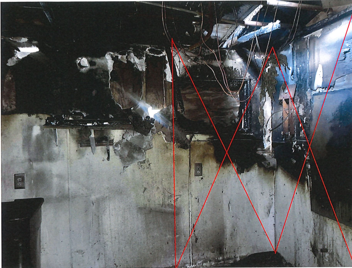
The exterior walls at the rear west corner should be rebuilt.
