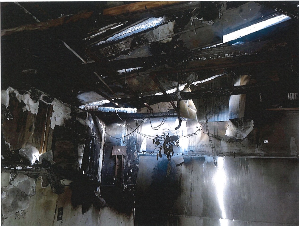
The structural fire damage was limited to the rear west corner of the kitchen.
