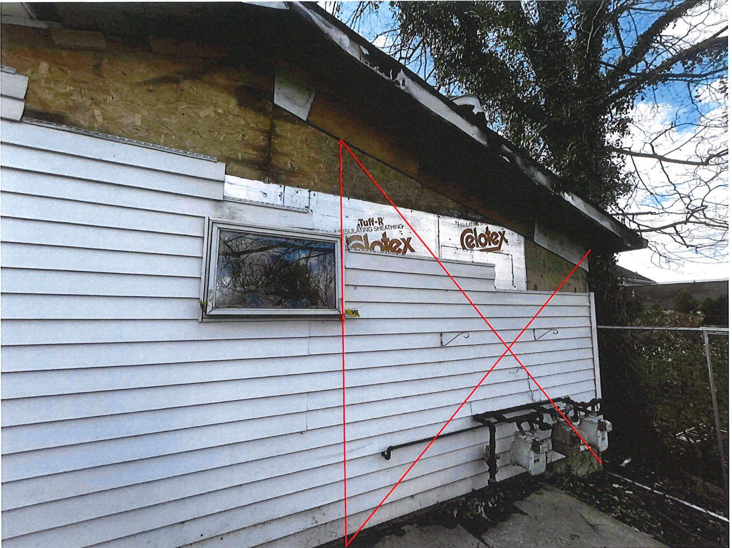
Most of the vinyl siding is intact indicating the limited damage from the fire.
